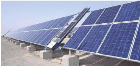
25KW PV System
